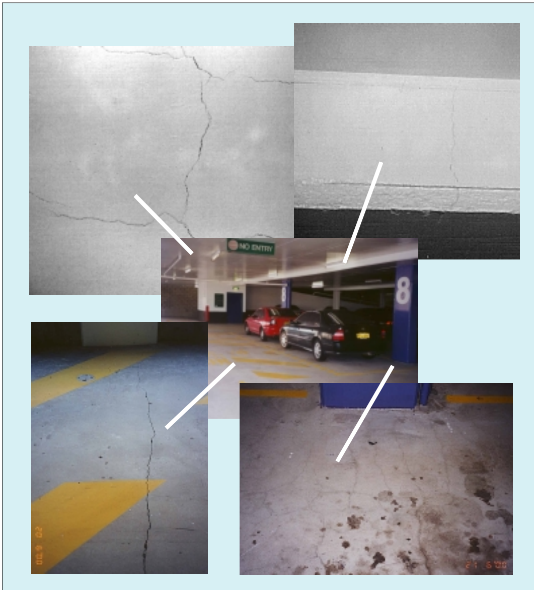
Figure 1.2 Avoidable Flexural Cracking in a Carpark
